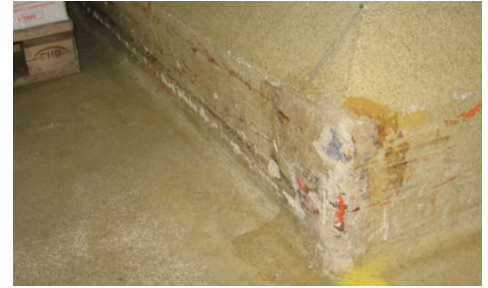
Example of concrete curb with resinous mortar. Signs of impact and damage. Concrete exposed to water will absorb and repel the covering resinous top layer and create a perfect harbor for bacterial growth.
